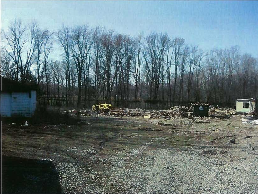
Date: 03/13/2012 Time: 9:55 a.m. Direction: south Photo by: Garrison Gross Exposure #: 003 Comments: demolition debris
