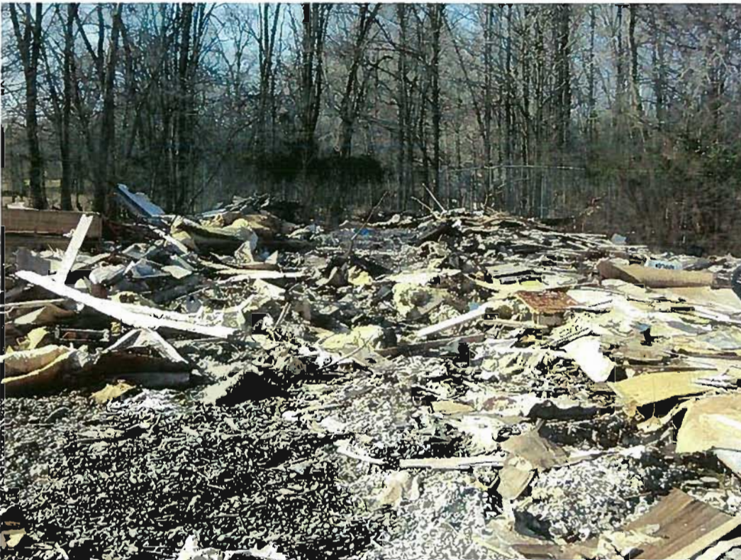
Date: 03/13/2012 Time: 10:00 a.m. Direction: south Photo by: Garrison Gross Exposure #: 008 Comments: demolition debris
