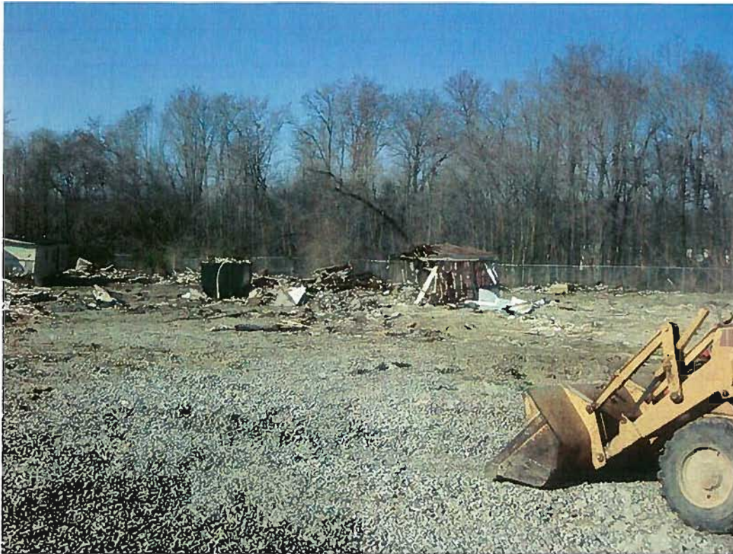
Date: 03/13/2012 Time: 9:55 a.m. Direction: southwest Photo by: Garrison Gross Exposure #: 001 Comments: demolition debris
